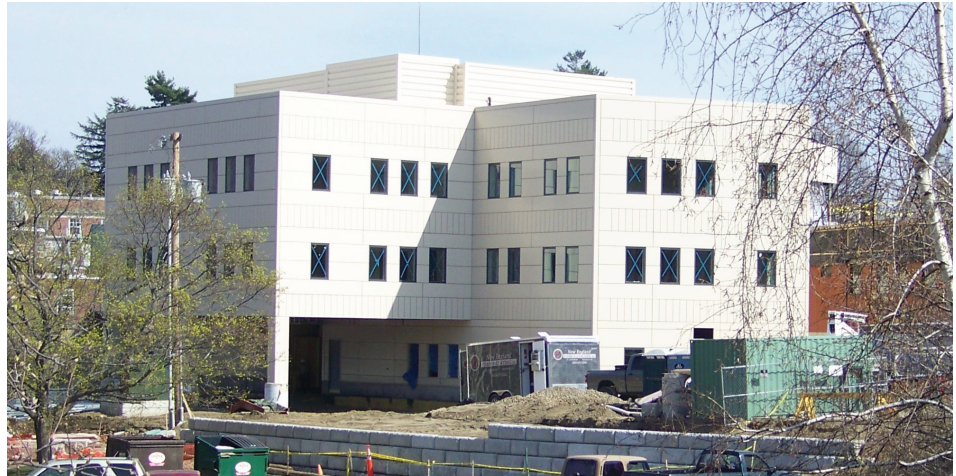
The new BMH Outpatient Building is nearing completion. This view shows the convenient, covered patient drop-off on the Maple Street side of the new complex which also accesses new parking spaces.
